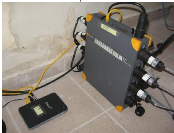
Fig. 2. Connecting measuring instruments Source: Author's
